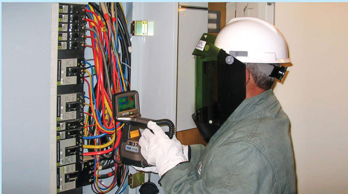
▲ Electrical Switchgear Testing
